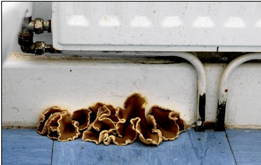
Figure 4 Fungus sprouting from skirting board area in the Balgaddy Development, built in Dublin in 2004. The fungus is a result of damp and condensation (Images from the Irish Times (Holland, 2011))
